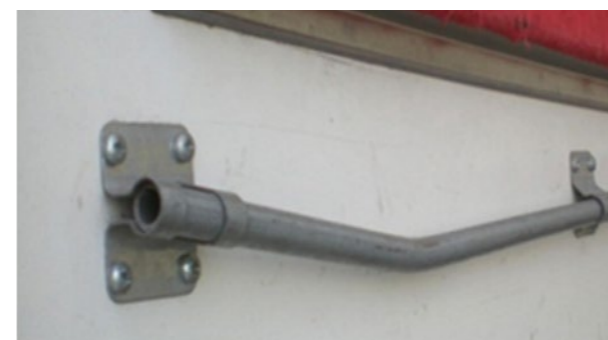
🔧 Upholstery and rods: Rods and upholstery damaged within economic repair
