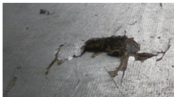
🔧 Flooring: Dents or perforations within economic repair
