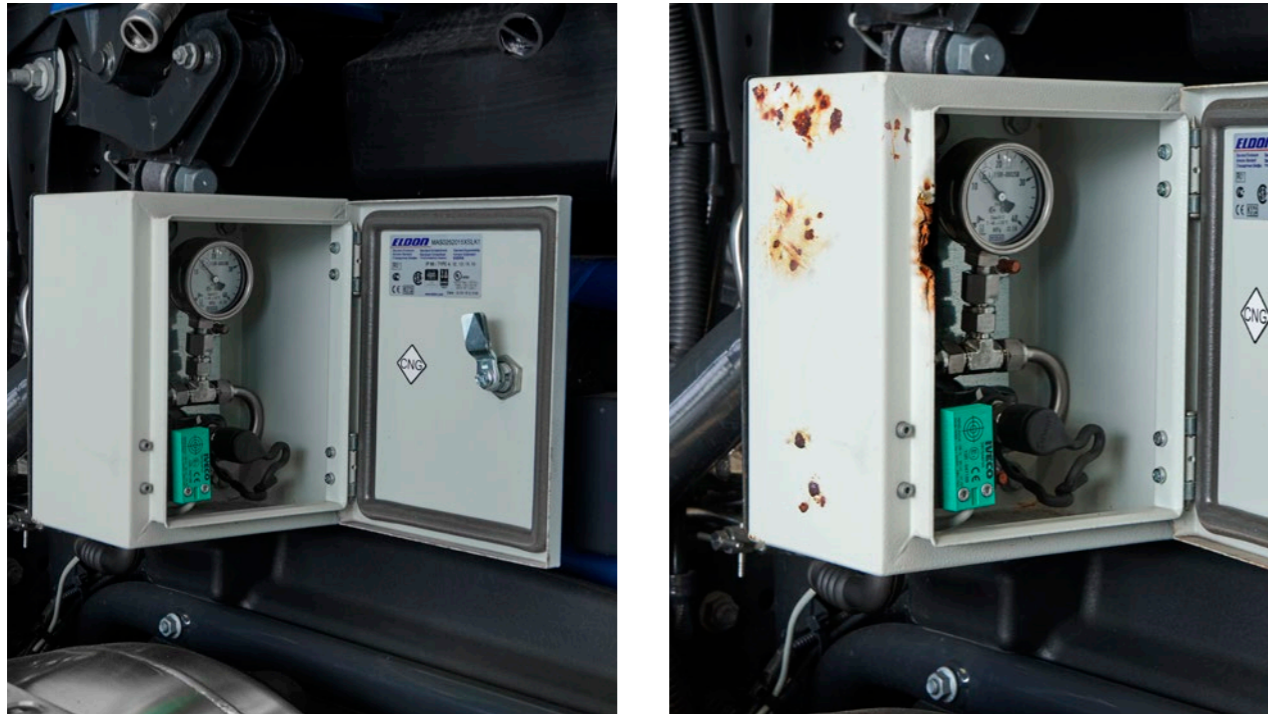
Rust on the fill receptacle protection box → note without charge for damage.
